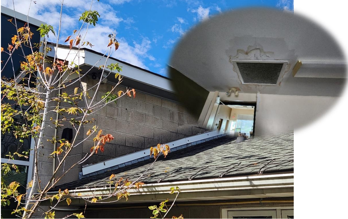
Addition Separating From Building – Attempt to improve flashing to stop water infiltration.
